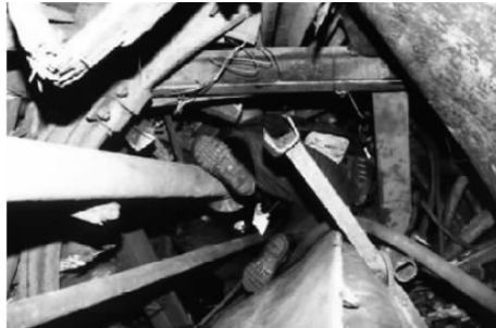
Fig. 2 Deep rock mass roadway support after impact ground pressure failure.
