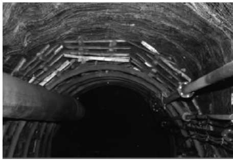
Fig. 1 Deep rock mass roadway support before impact ground pressure failure.
