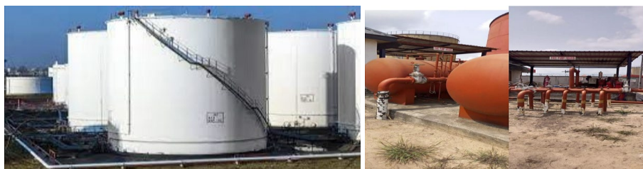
Fig. 3 Typical tank farm and fire pump station.
